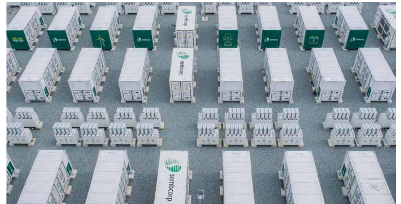
Sembcorp Banyan Energy Storage System on Jurong Island, Singapore
