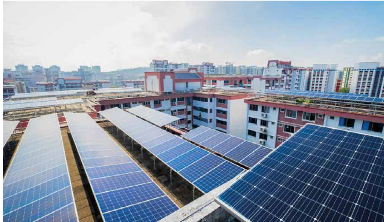
Solar photovoltaic (PV) systems installed on top of housing blocks as part of Singapore's SolarNova programme
