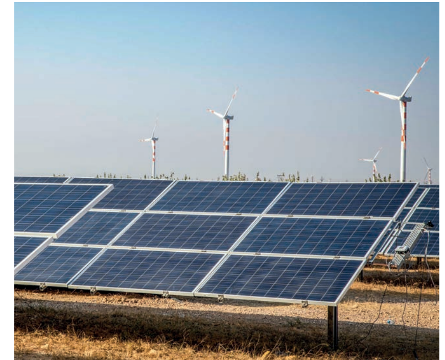
Sembcorp's hybrid renewables project in Rajasthan, India
